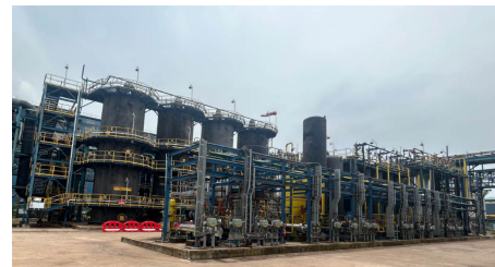
PyroGenesis' Coke Oven Gas and Hydrogen Extraction System at Tata Steel, Kalinganagar, India
