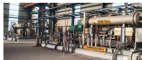
Water-Injected Compressor Units in Use at Tata Steel, Kalinganagar, India
