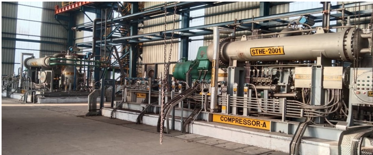
Image 2: Water-Injected Compressor Units in Use at Tata Steel, Kalinganagar, India
