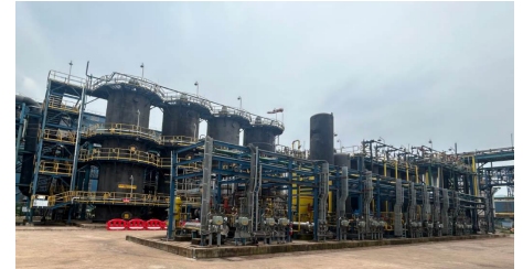
PyroGenesis' Coke Oven Gas and Hydrogen Extraction System at Tata Steel, Kalinganagar, India
