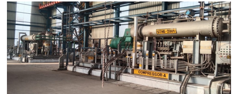
Water-Injected Compressor Units in Use at Tata Steel, Kalinganagar, India
