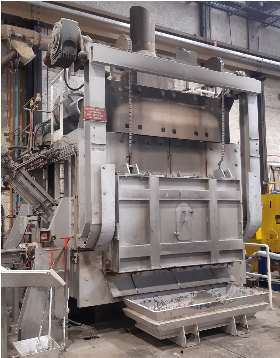
Image 1: reverberatory melting furnace in use at one of Constellium's aluminum facilities.
