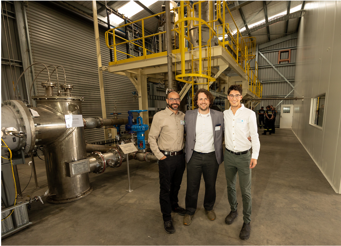
Image 4: PyroGenesis' engineering team José Urbina, Jean-René Gagnon, and Aidan Moir, stand in front of PyroGenesis' all-electric plasma-based SPARC™ system, at the opening of New Zealand's National Refrigerant Destruction Facility. Photo Credit: Jamie Troughton/Dscribe Media.
