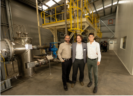
PyroGenesis' engineering team José Urbina, Jean-René Gagnon, and Aidan Moir, stand in front of PyroGenesis' all-electric plasma-based SPARC™ system, at the opening of New Zealand's National Refrigerant Destruction Facility. Photo Credit: Jamie Troughton/Dscribe Media
