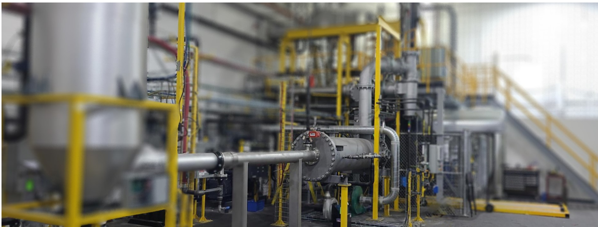
Figure 1- Picture of PyroGenesis' Gen3 PUREVAP™ Quartz Reduction Reactor (QRR) pilot plant
